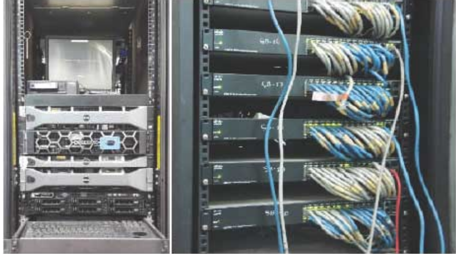
Server and Network Infrastructure
